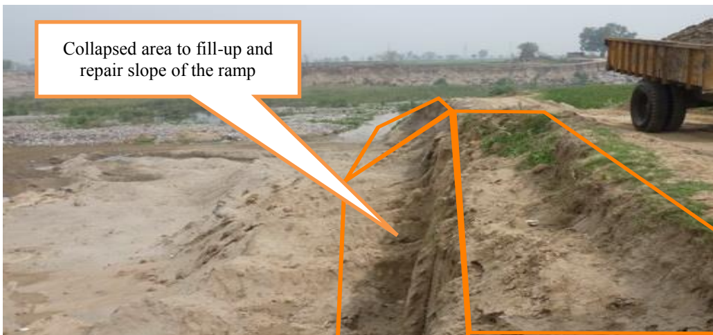
Photo 5.3.1 Collapse of Gondlanwala Landfill Site
