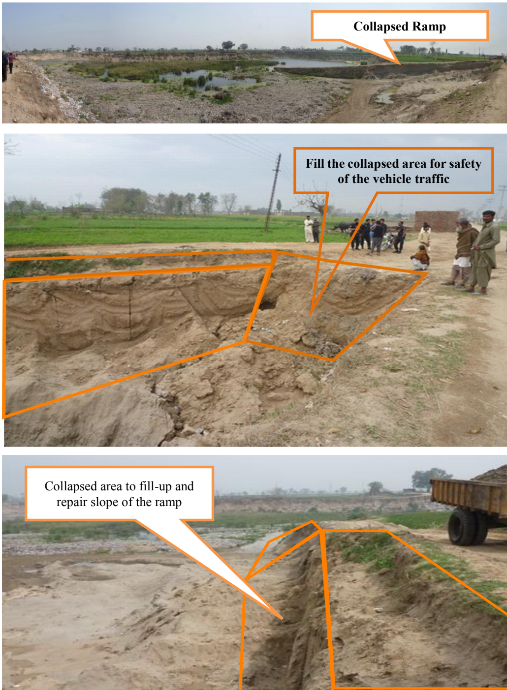
Photo 4.5.1 Collapse of Gondlanwala Landfill Site
