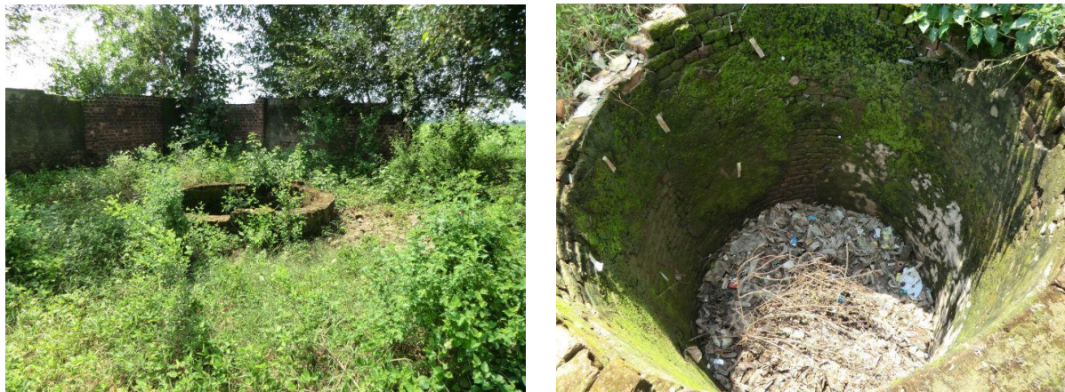
Photo I.2.3 Pit for Risk Waste at BHU
