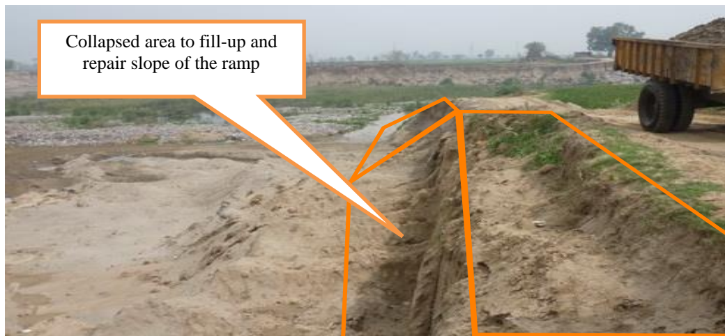
Photo C.4.1 Collapse of Gondlanwala Landfill Site
